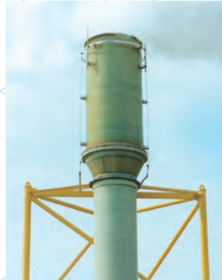
Chimney swirl droplet separator at BASF
