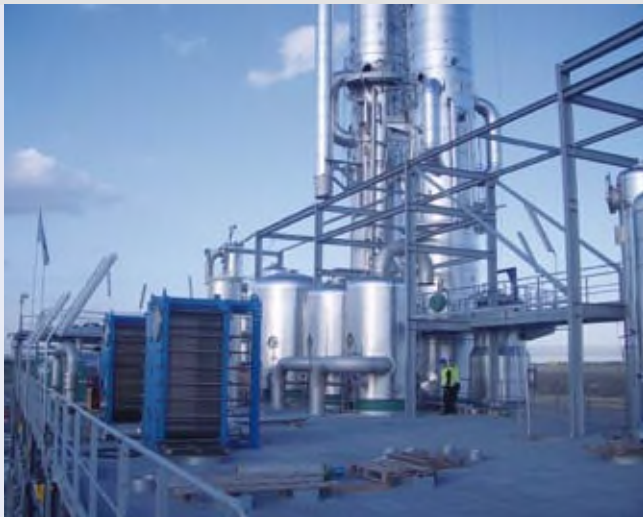
Condensation of bioethanol.
