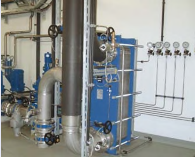
Hydraulic oil cooling in power plant.
