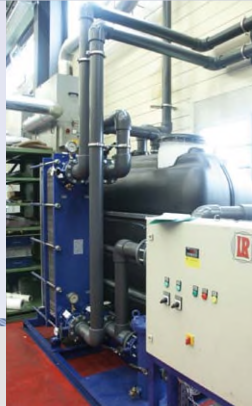
Cooling of lubricating oil for extruding presses.
